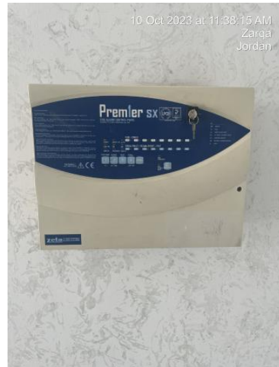
Firefighting control panel.jpeg
